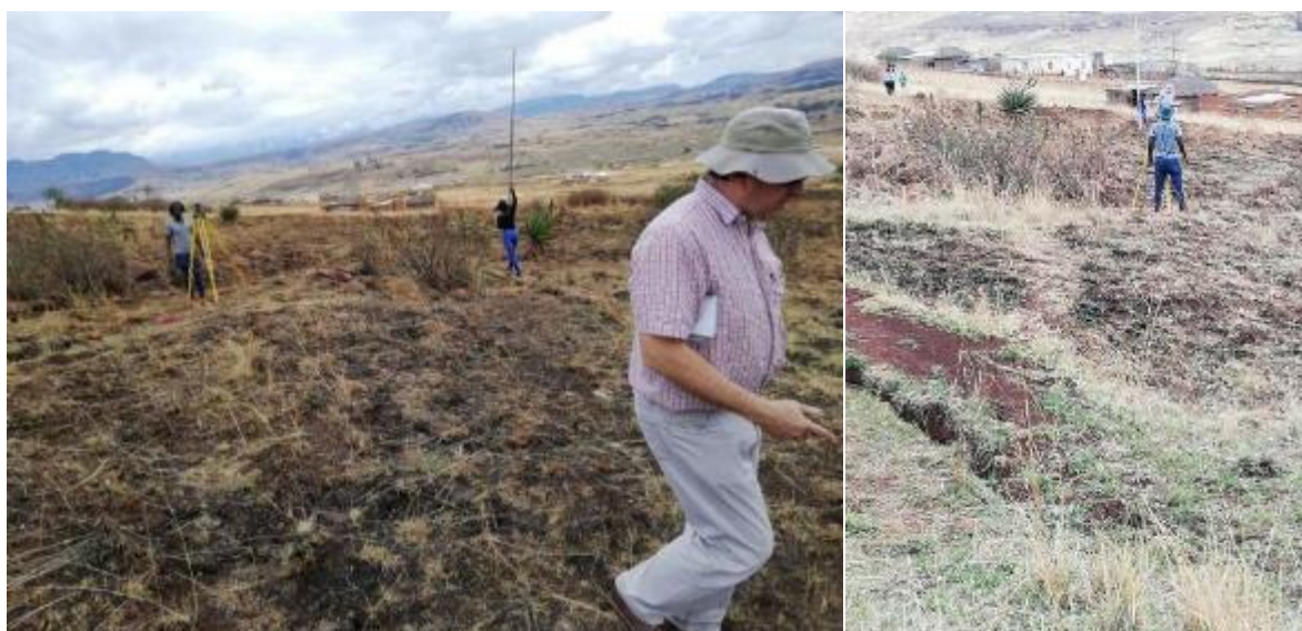
Figure 43: Left; Measuring the gradient for the main pipeline using a dumpy level. And Right; adjusting the line for the pipe to avoid some of the larger dongas and rough terrain, while keeping it on an even gradient.
