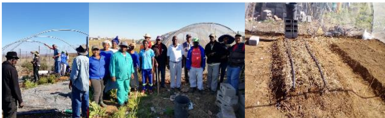
Figure 19: Above Left; learning group members constructing the tunnel, Centre; the final product and Right; construction of the deep trench beds with installation of the drip irrigation kit at Xhukwane
