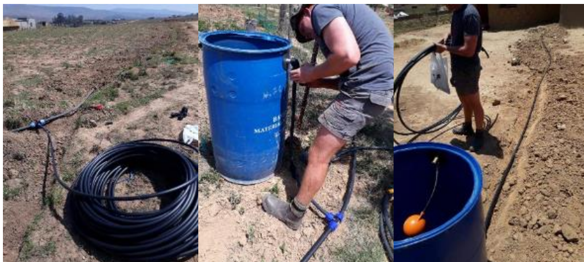
Figure 47: Above Left to Right: Laying the piping along the edges of the fields, with branches towards the different homestead; fitting the inlet pipes to the 200l drums and installation of a float valve in each drum.
