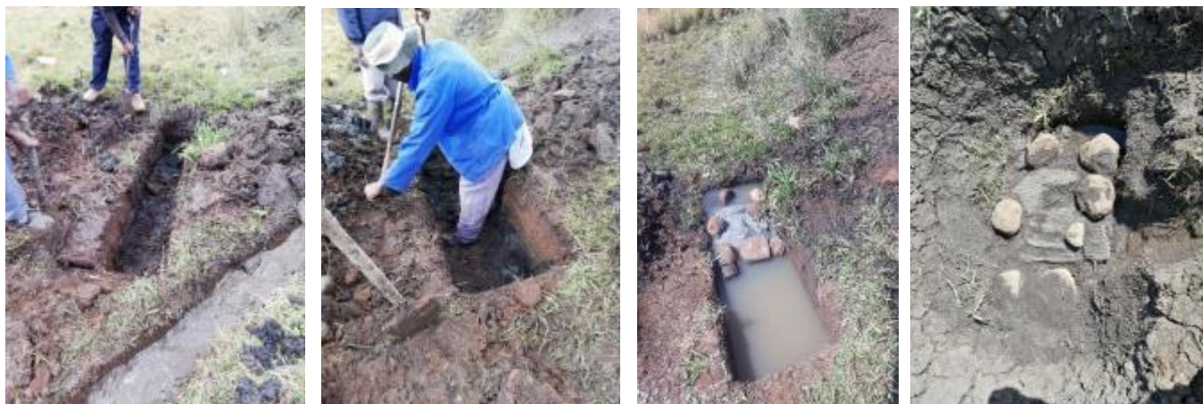
Figure 42: From Left to right; Starting on the trench for the slotted pipe, below the spring and pond, deepening and widening this trench to 50cm x50cm x 1,2m), the trench with slotted pipe installed in a bed of gravel, covered by shade cloth and rocks with a small furrow leading water from the spring to this trench and the trench damaged by livestock before it could be properly covered and closed.
