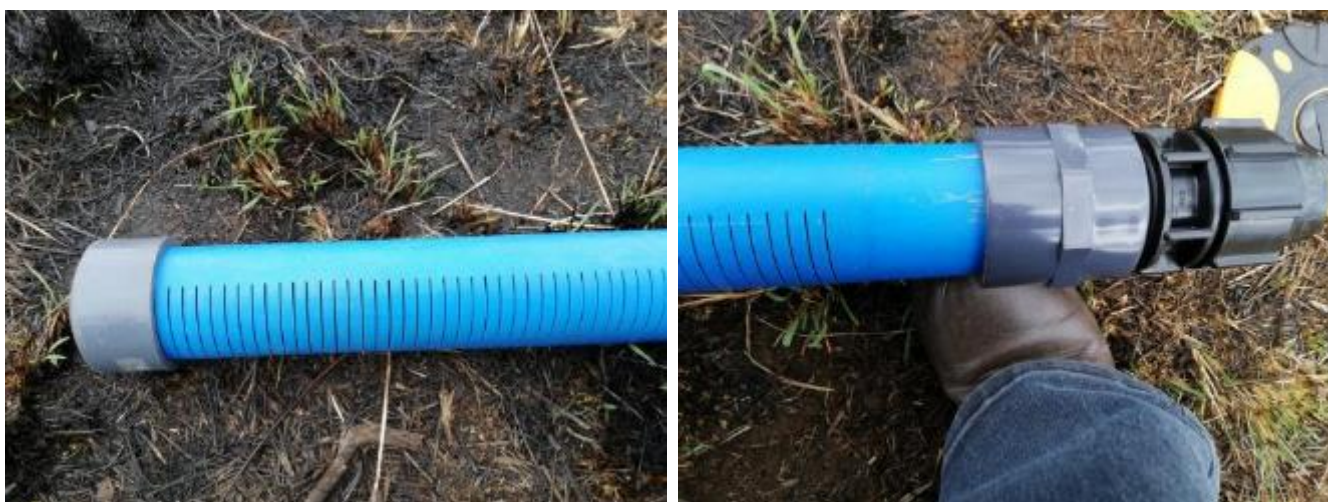
offtake of water from the spring and Right; the fittings linking this slotted pipe to the main pipe (50mm HDPE) (from Chris Stimie- RIEng)
