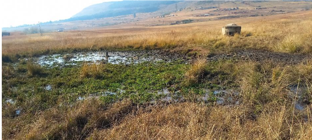
Figure 3: The old, protected spring with leaking header tank and inaccessible tap.
