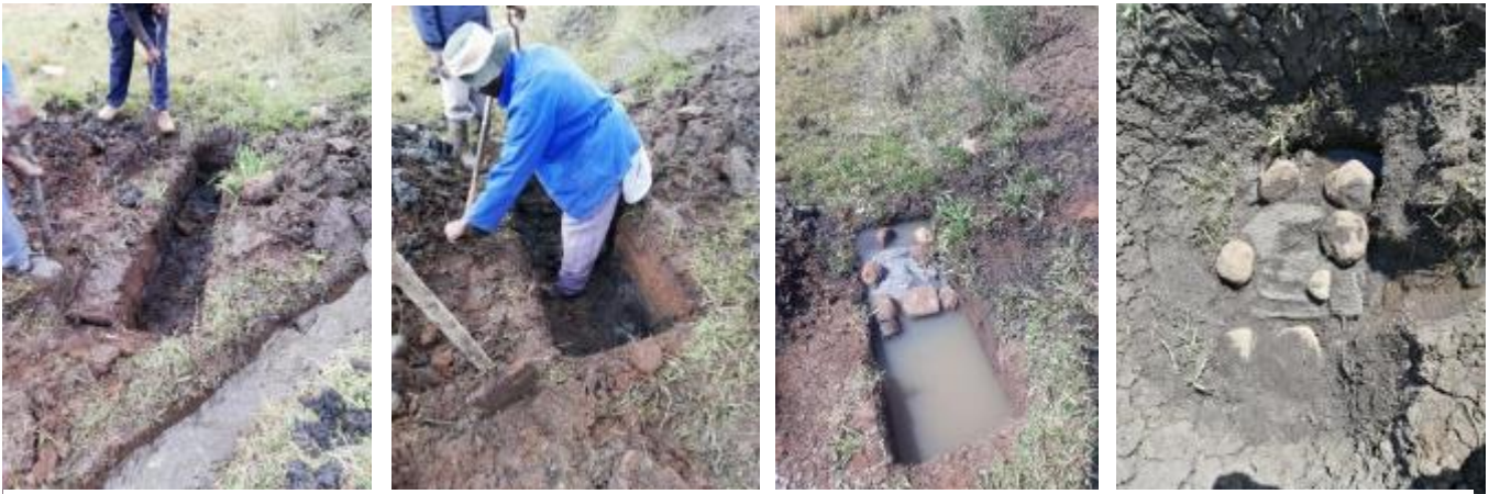
Starting on the trench for the slotted pipe, below the spring and pond
