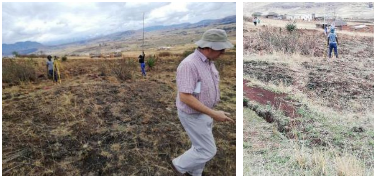
Figure 18: Left: measuring the gradient for the main pipeline using a dumpy level. Right: Adjusting the line for the pipe to avoid some of the larger dongas and rough terrain, while keeping it on an even gradient.
