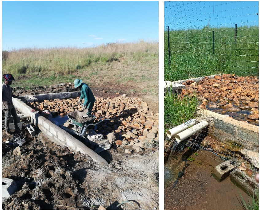
Figure 13: Below Left and Right: The 2 x 5000l header tanks at installation and recently in Feb '23 – also fenced.
