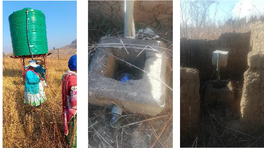
Figure 1: Above Left: the header tank for the SAPPI borehole. Centre: the pump for the borehole and right: The enclosure built for the pump and electrical box.
