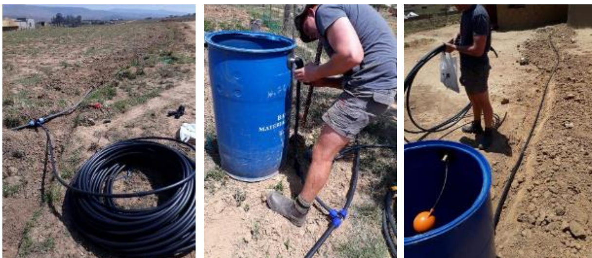
Figure 22: Left to right: Laying the piping along the edges of the fields. Pipe branches towards the different homesteads. Fitting the inlet pipes to the 200 L drums. Installation of a float valve in each drum.
