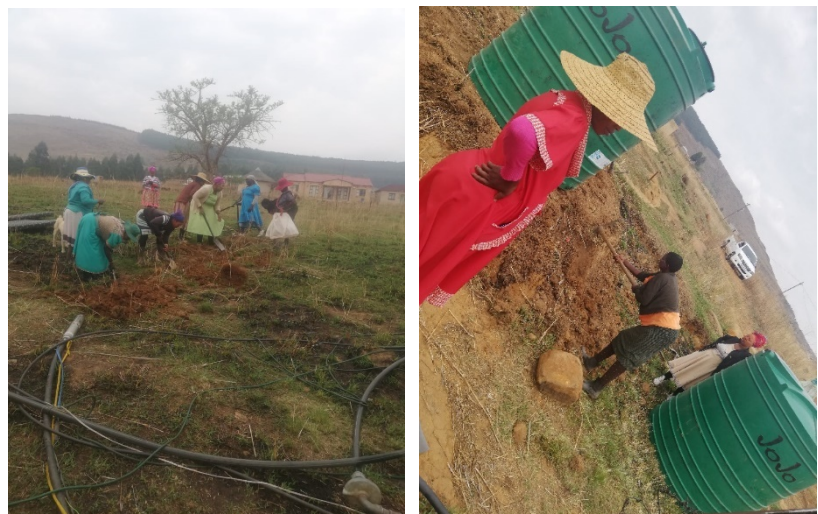
Figure 7: Right: The piping from the borehole yield testing is shown in the foreground. And Far right: Community members levelled platforms for the two extra JoJo tanks so that water could be stored temporarily for the community.
